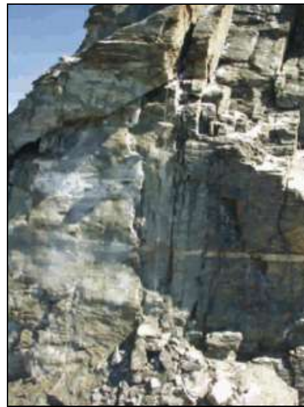
Fig. 7: Rock fall starting zone on the Matterhorn in summer 2003. On the left side ice is still visible on the surface of rupture.
